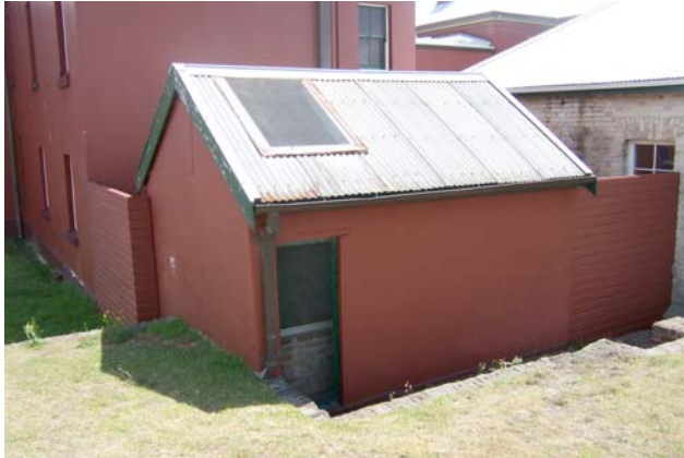
Fig. 4. 2 View of Store Room displaying the mesh openings on the roof and east facade.
