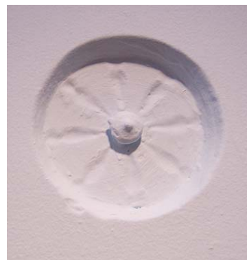
Fig. 2.3 (Right): Vent as seen from interior – note plaster has been used to fill vent openings.
