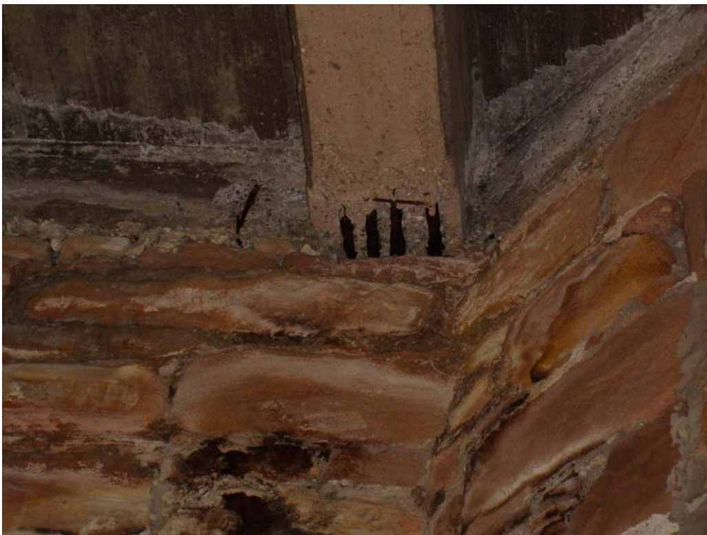
Fig. 4 The west end of the hanging concrete beam under concrete slab roof, showing the exposed and rusting reinforcing rods. (Photograph by Sheppard, October 2006)
