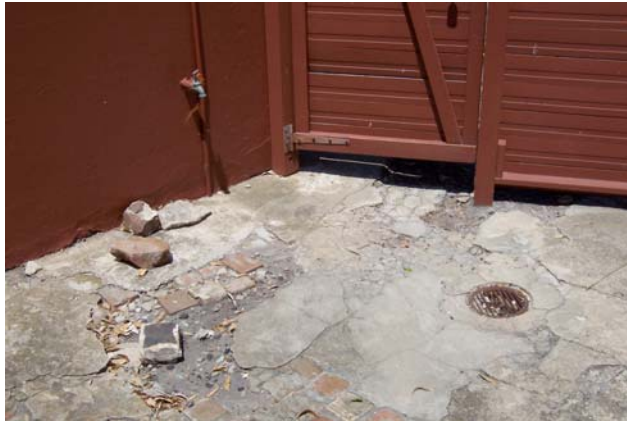
Fig. 5.10 Uneven and deteriorated ground surface in the courtyard area.
