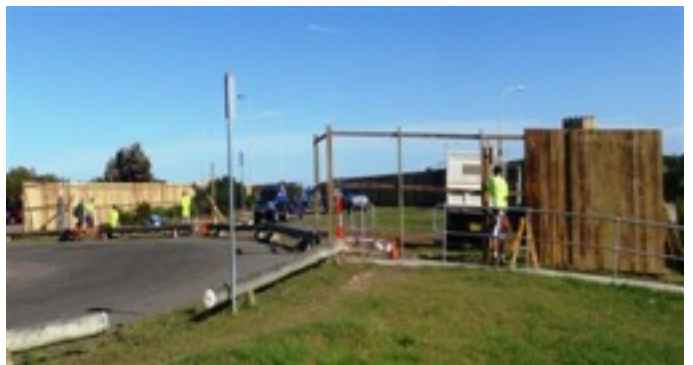
(Fencing off at La Perouse Winter 2009–Winter 2010 for Botany Bay Cable construction)
